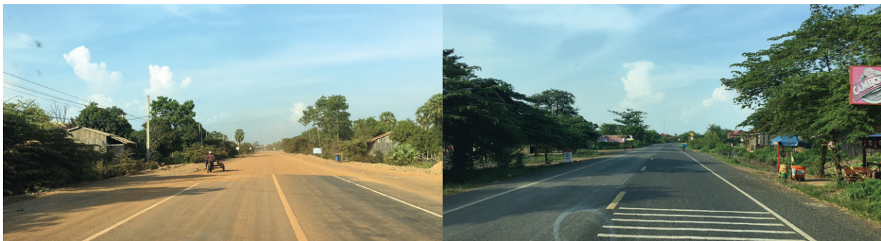
Left and right photos: Sections of Kratie–Stung Treng . Two lane double bituminous surface treatment road.
