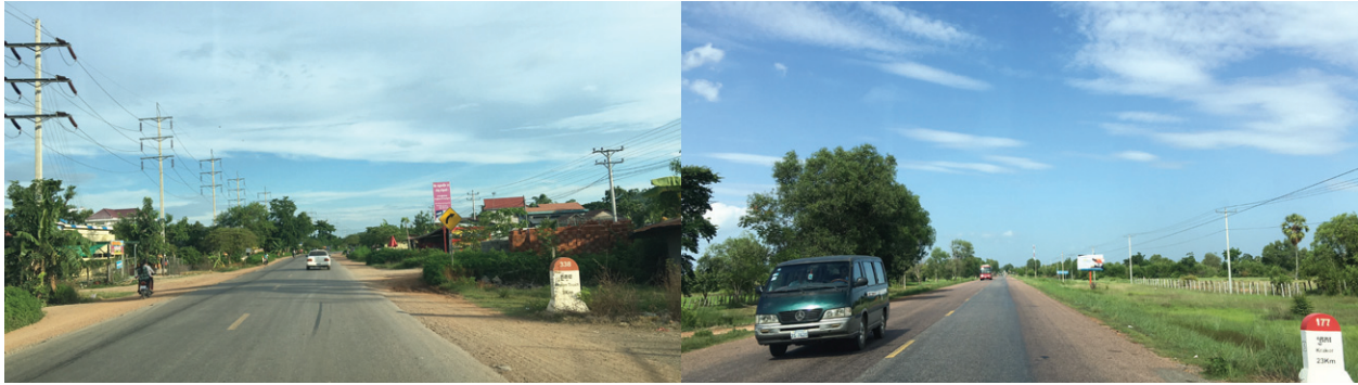
Left: Sisophon–Battambang . Right: Battambang–Kampong Chnang . The pictures show the existing road condition before the upgrading and widening through a loan from Japan.
