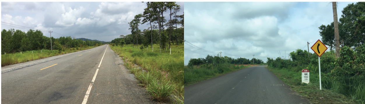
Left: O Pong Mon–Bang Lung. Condition of road in NR No. 78. Right: Bang Lung–O Yadav Border. Part of the 68 km road from Bang Lung to O Yadav in the Cambodia-Viet Nam border.
